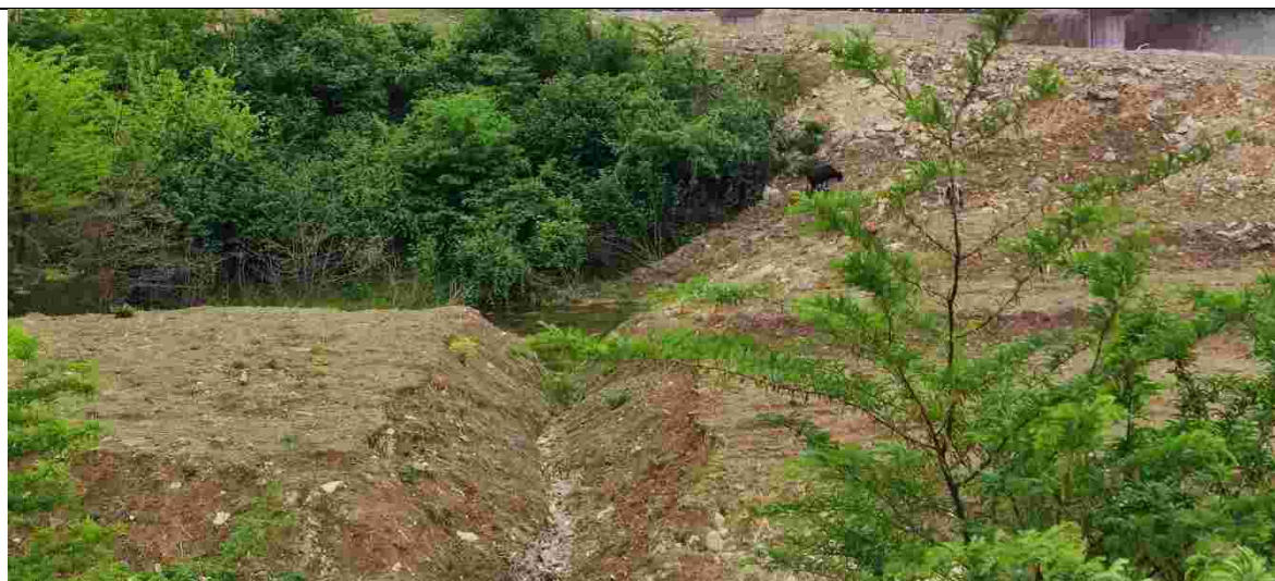
Drainage Issue for Spoil Disposal Site No: 3 (Panoramic View, May 2024)
